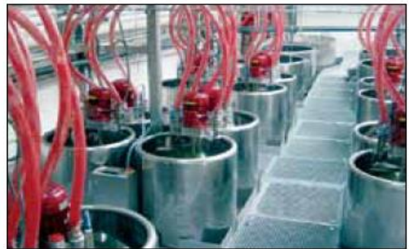
Color kitchen with automatic thickener and water dosing
