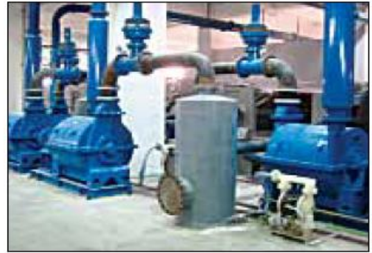
Vacuum pumps of washing unit
