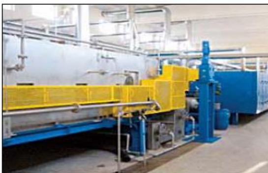
Horizontal steamer, washing unit and dryer
