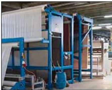
Unrolling, J-box, lint removal, pre-steamer, edge guiding and pull roller
